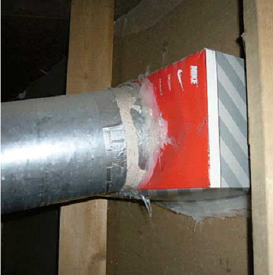
The latest in designer outside air plenums
